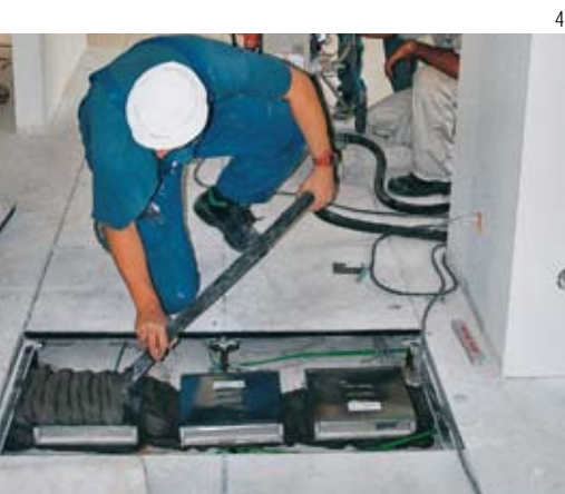
4 The topic of fire protection is becoming increasingly important. Here, a distribution shaft is being filled.
