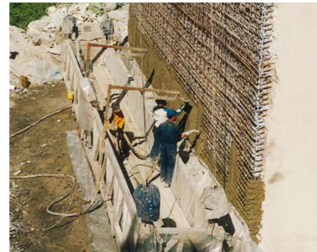
They are also extremely suitable for large jobs, as here for the concrete refurbishment of a motorway bridge in Italy.
